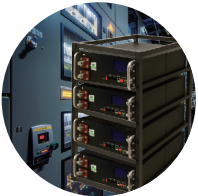
Rack-mounted Energy Storage
